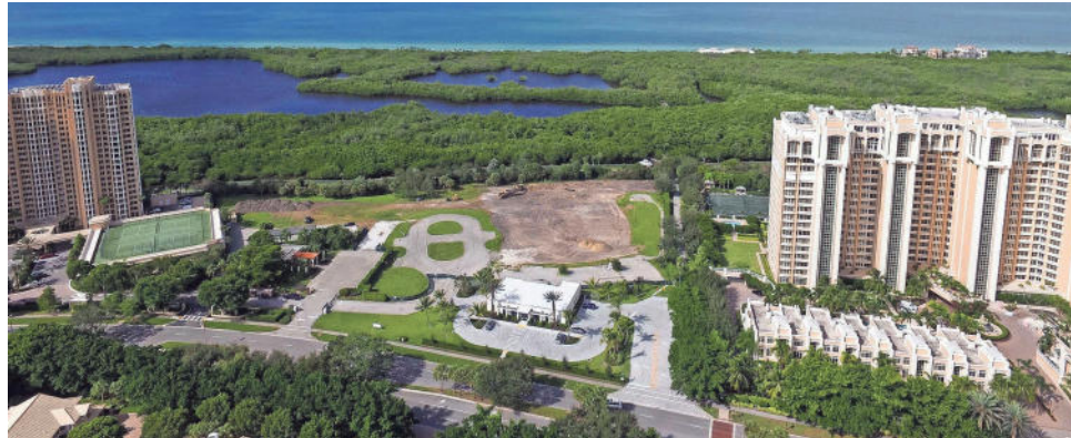
Infrastructure and site development is underway for Mystique, a new luxury high-rise by Gulf Bay in Pelican Bay.
