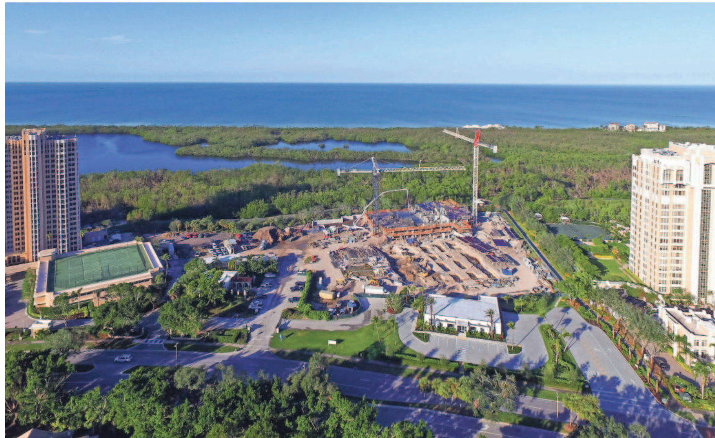
The first residential floor has been poured for Mystique, a 20-story tower in Pelican Bay. SUBMITTED
